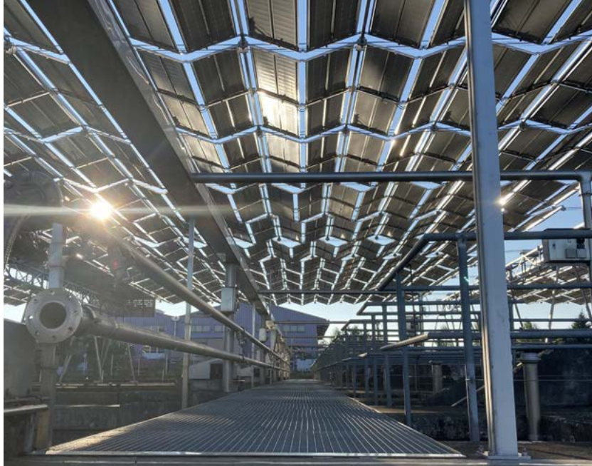
Morgental solar power plant (CH)
